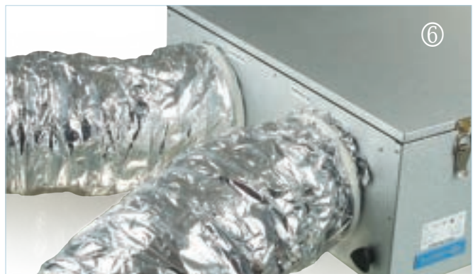
Heat-insulated air ducts have reliable connection to the air handling unit spigots.
